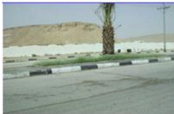
Green Zone Cracks
