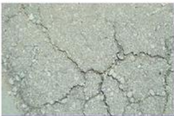
Rut Ridge Cracks
